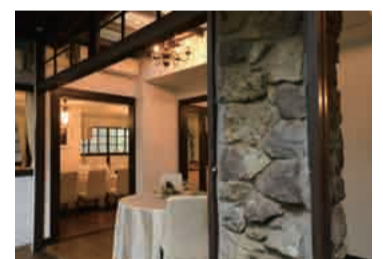
Some earthquake reinforcement has been carried out for the building, and the stones forming the pillar are the same as ones put in place when the building was completed.
