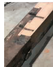
A cross-section showing where old material has been integrated with new material, using the kanawa-tsugi technique. If used at the base of a pillar, when the material is stressed from the right, left, front or rear, it deforms based on the direction of the stress, and returns to its original shape in a flexible manner.
