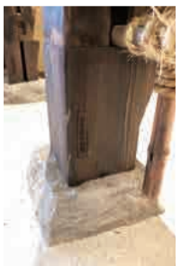
The delicate beauty of the takekomai foundations. New material has been added to the lower section to maintain its integrity, and there is an engraving that says, "Repaired in the 3 rd year of Reiwa."
